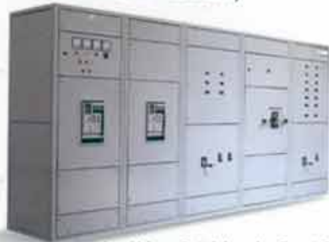
Low Voltage Switch boards - Type MF
